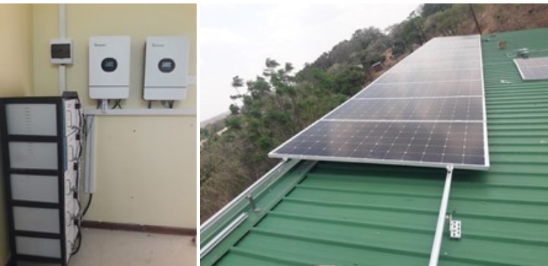
(Pictures while work was in progress) Two maternity ward buildings are now solar powered
